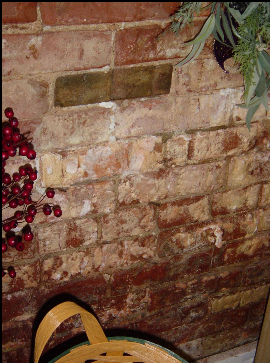
Damp mossy interior walls
