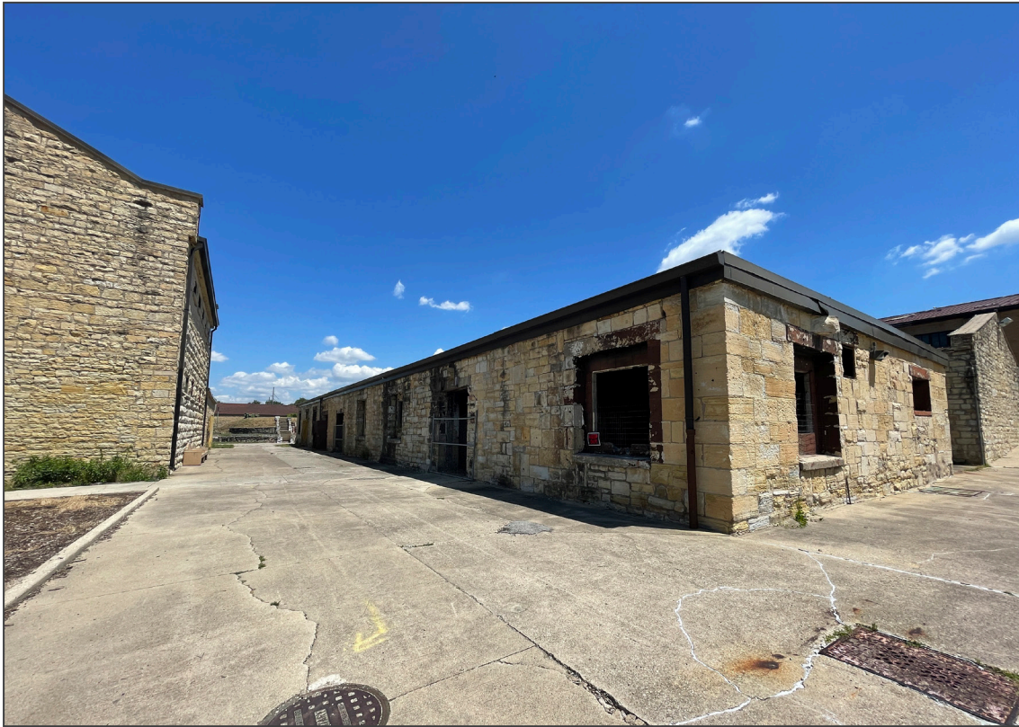
28. Harness Shop (#23), south and west elevations, view northeast. Partial view of Separate System Prison (#15) at left.
