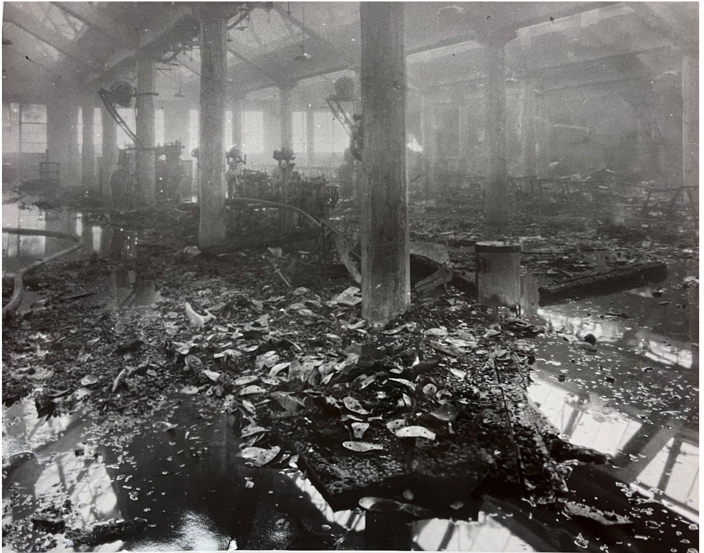
Figure 35: Damage to the shoe factory at Joliet Penitentiary after the 1931 riot (Joliet Area Historical Museum)
