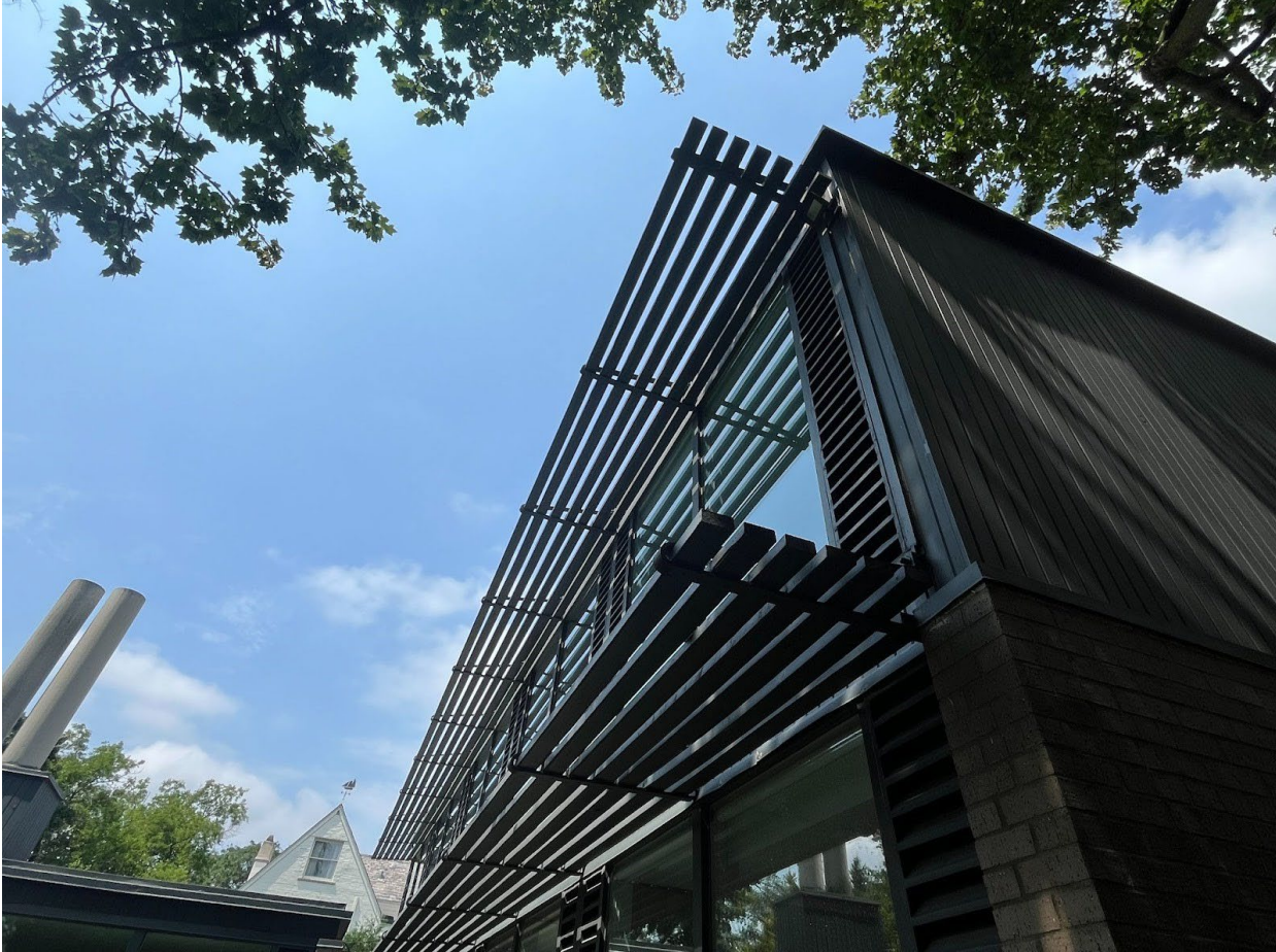
Detail of Sunshades on North (Front) Wing South Elevation, camera facing northwest
