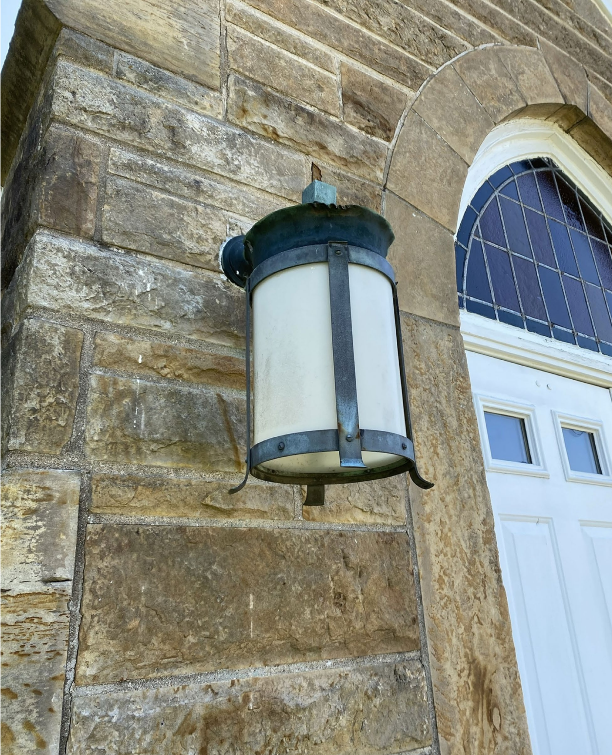
Photo 5: Original lighting near front entrance, looking northeast
