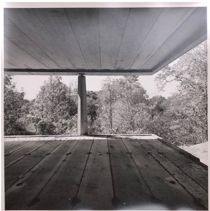
Figure 7: The Rockwell House, column and roof plate, construction photo, Olympia Fields, IL (1963). Brenner-Danforth-Rockwell, architects. Tapered concrete column supports a "floating" concrete roof. Image: Richard Nickel. Ryerson and Burnham Art and Architecture Archives, The Art Institute of Chicago.
