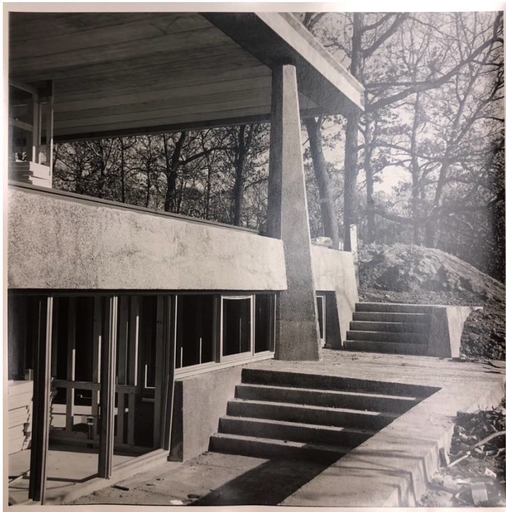
Figure 6: The Rockwell House, south elevation, construction photo, Olympia Fields, IL (1963). Brenner-Danforth-Rockwell, architects. Image: Richard Nickel. Ryerson and Burnham Art and Architecture Archives, The Art Institute of Chicago.
