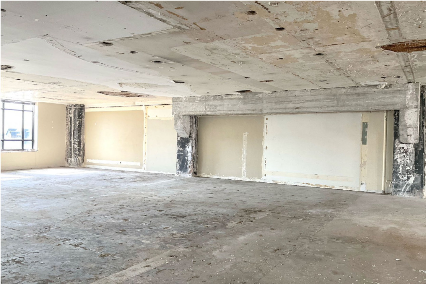
Photo 13 of 14: Oak Leaves Building, interior, 4th floor, looking southwest, showing additional concrete structure for building connection support
