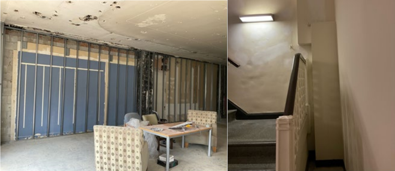
Photo on the right is taken from the Marshall Field side at the 3 rd floor landing and shows boxed-out areas, presumably to hide and clean up the structure from a previous connection here.
