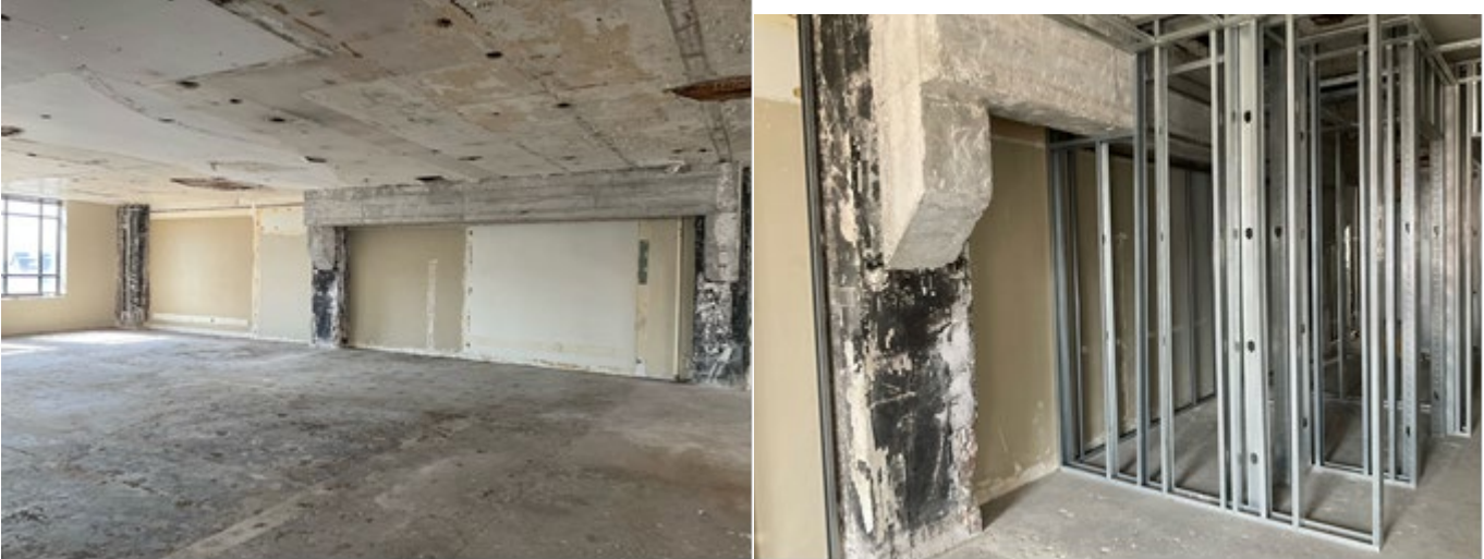
Figure 2: Additional concrete structure on the west wall on the 4th floor of the Oak Leaves Building, presumed to have been added to frame and support a previous opening and connection.
