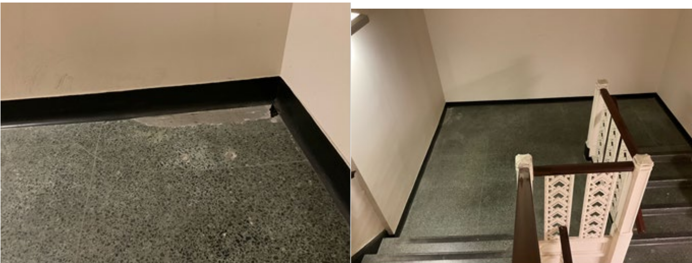
Close-up (left) and looking down on the landing from further back (right).
