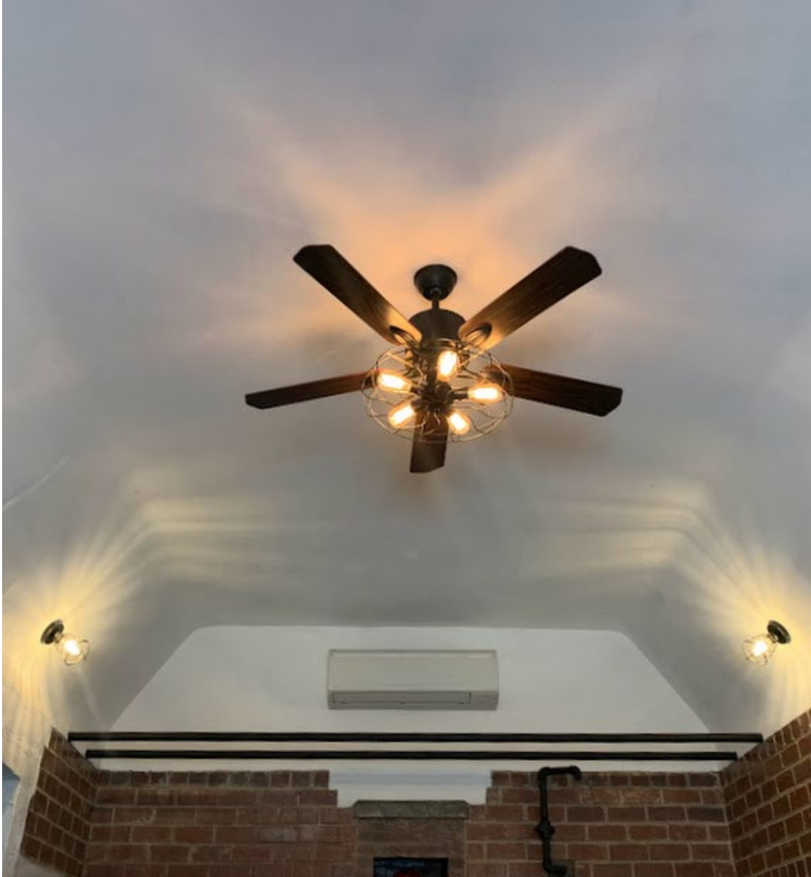
Photo 8 of 11: Service bay Ceiling repair, Original light fixture locations remain, camera facing south.
