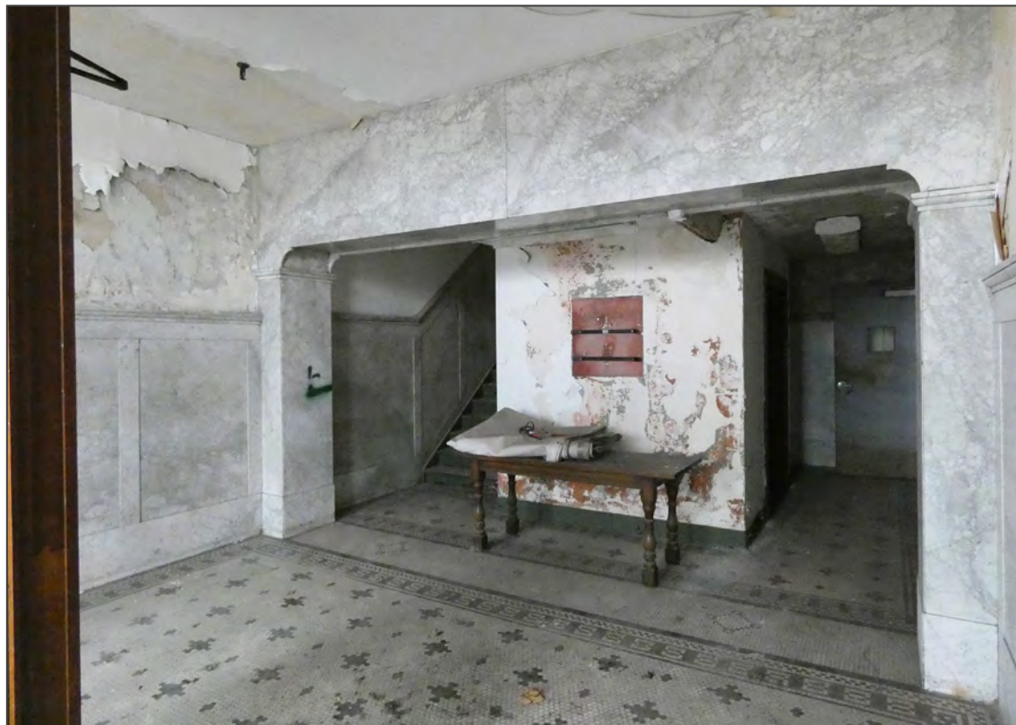
Photo 8. Ground floor entrance lobby, looking north at southwest stairwell (left) and passenger elevator (right).
