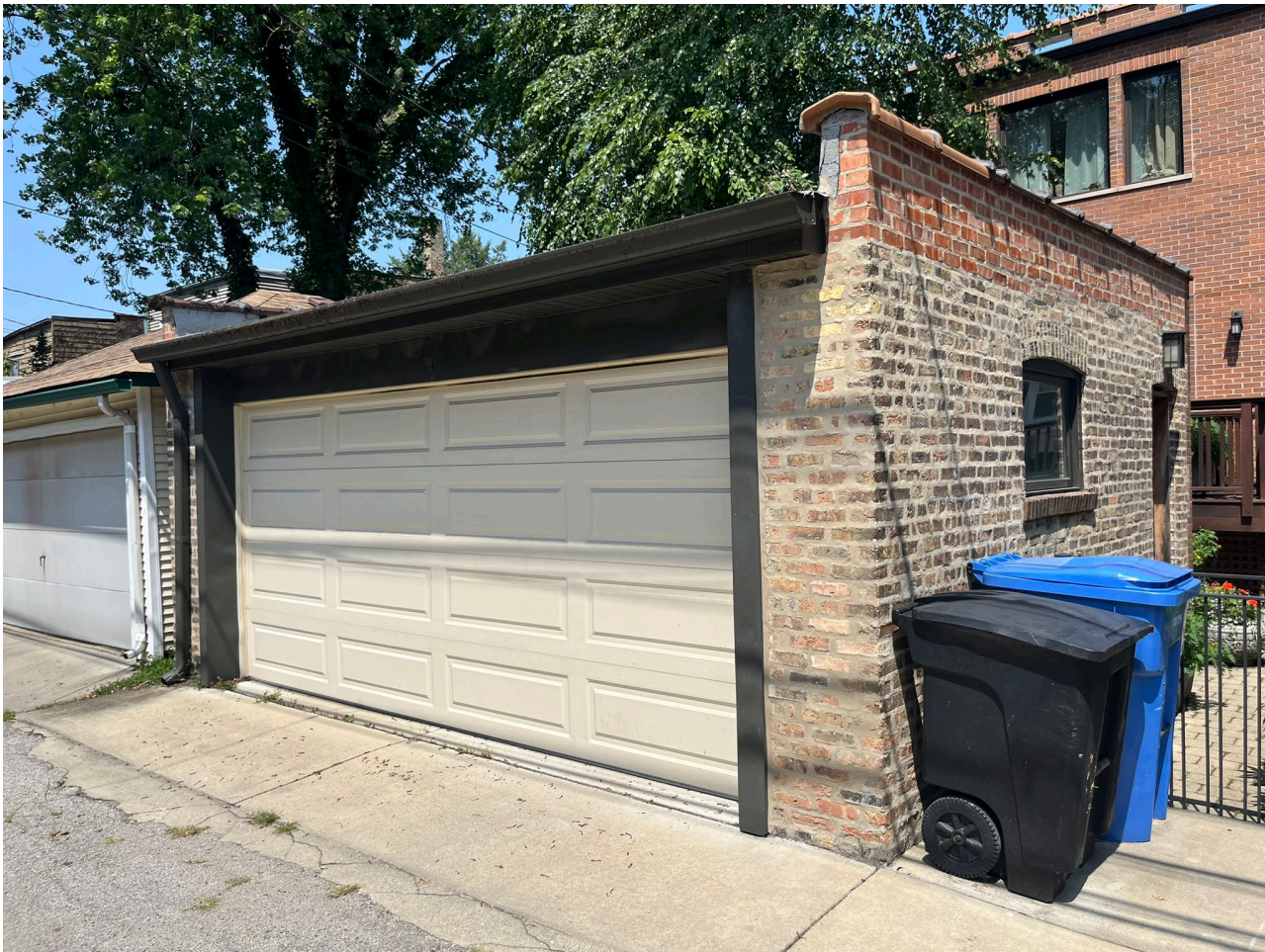
IMAGE 17: 1319 W. Norwood Avenue: Representative contributing garage with common brick walls and flat roof with parapet.
