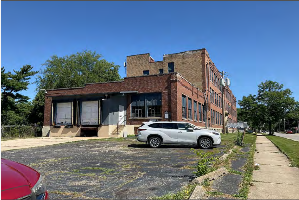
6. South and east elevations, 1917 south addition (middle) and 1912 block (right), facing northwest
